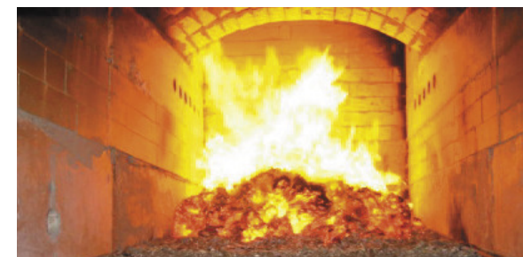
View into the combustion chamber with dome-shape brick refractory
