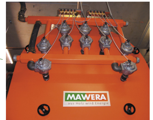
Add-on soot blower for cleaning heat exchanger
