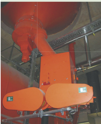
Silo reclaim system PS series feeding into a switch box
